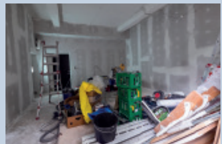
Kuratorisk Aktion carried out the renovation work of CAMP together with staff and asylum interns from Trampoline House. Photos: CAMP
